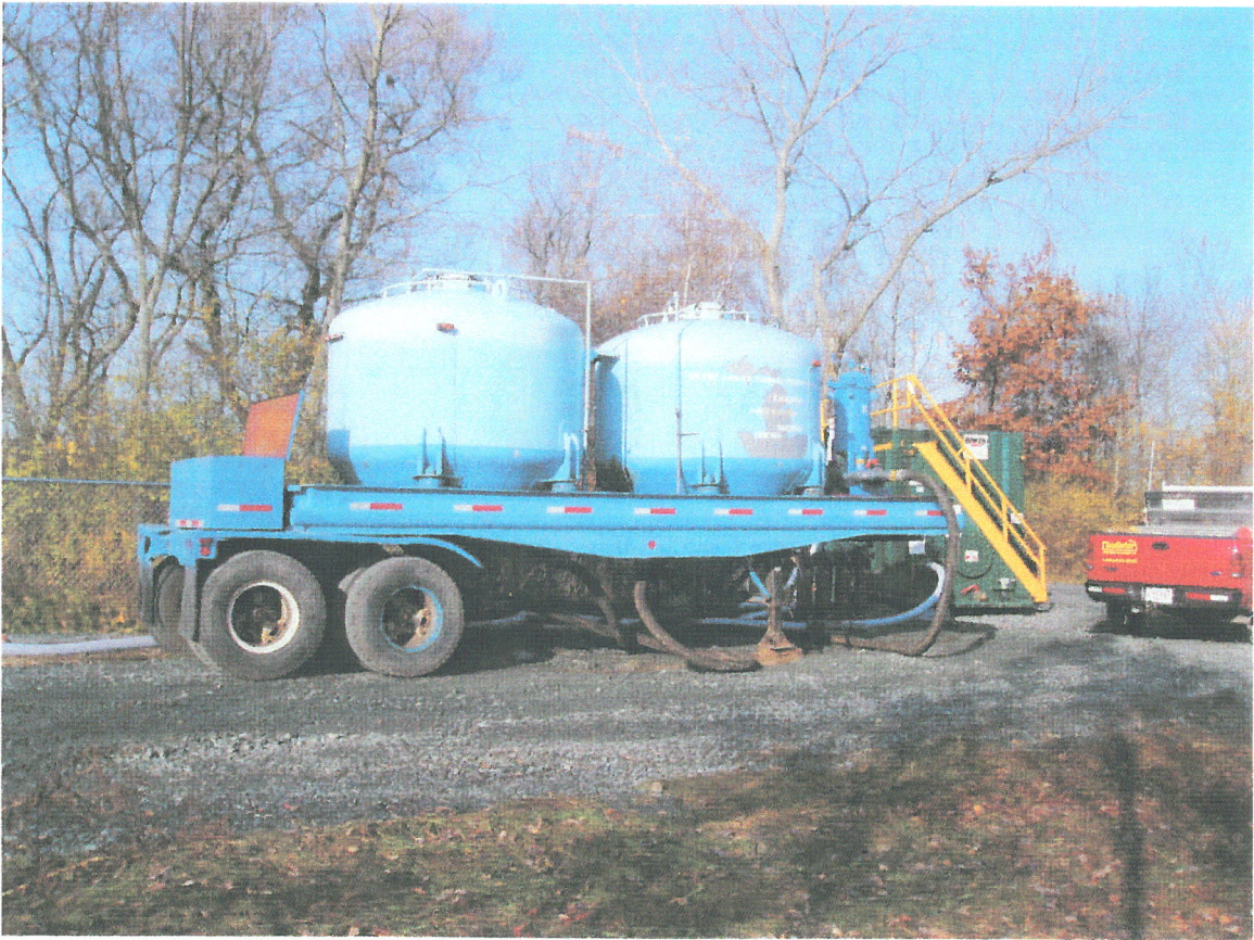
Water Treatment System: Activated Carbon Tanks
