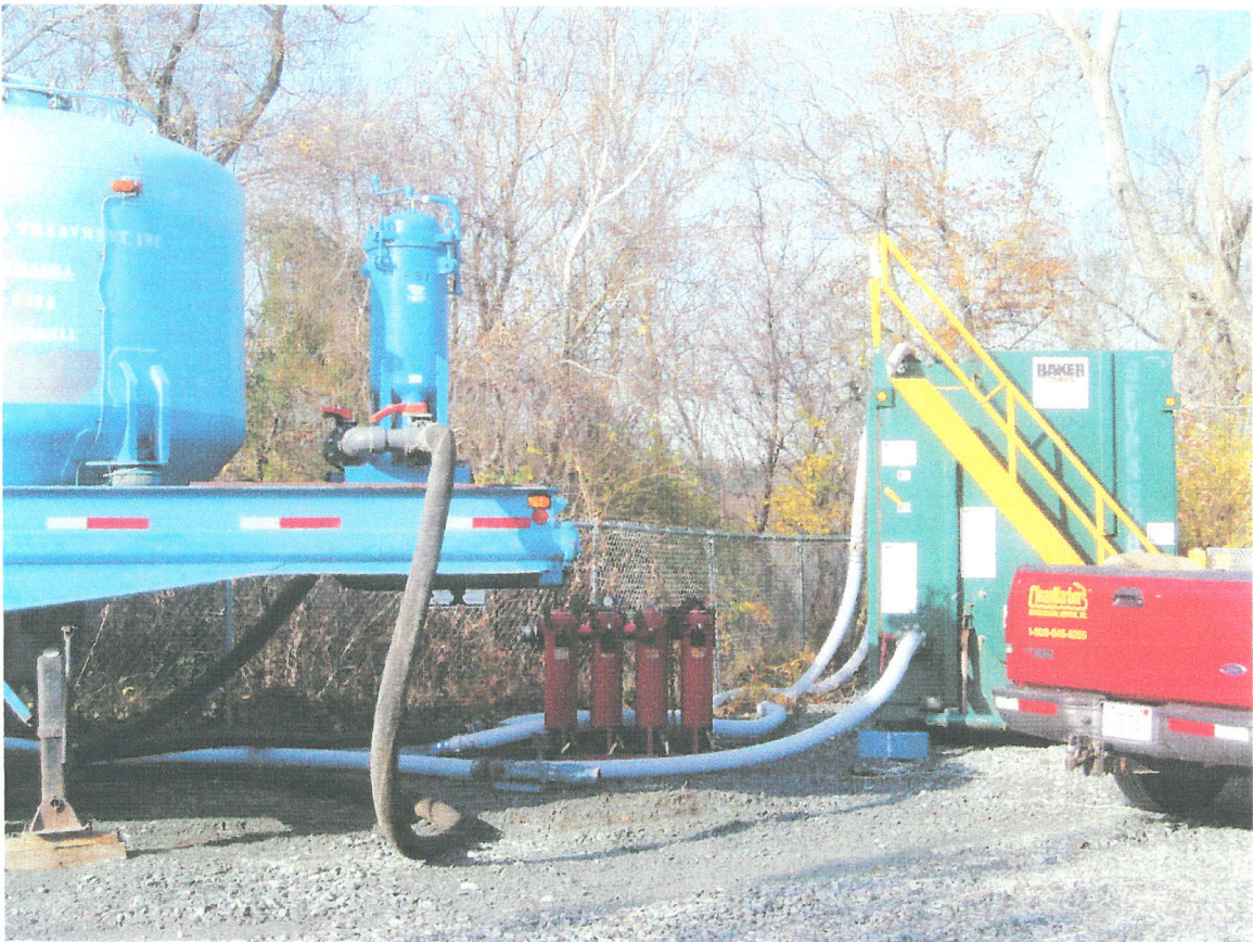
Water Treatment System: Frac Tank and Bag Filters
